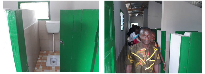
Renovated Bathroom of Aburi Girls SHS Showing Sample Pictures of the Squatting Toilet
